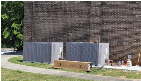
The second new HVAC unit made it on the slab this week.
